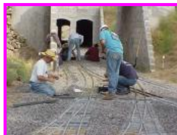
The Kitsap gang hard at work installing some more of those great ground throws, this time down in the South Portal area.
